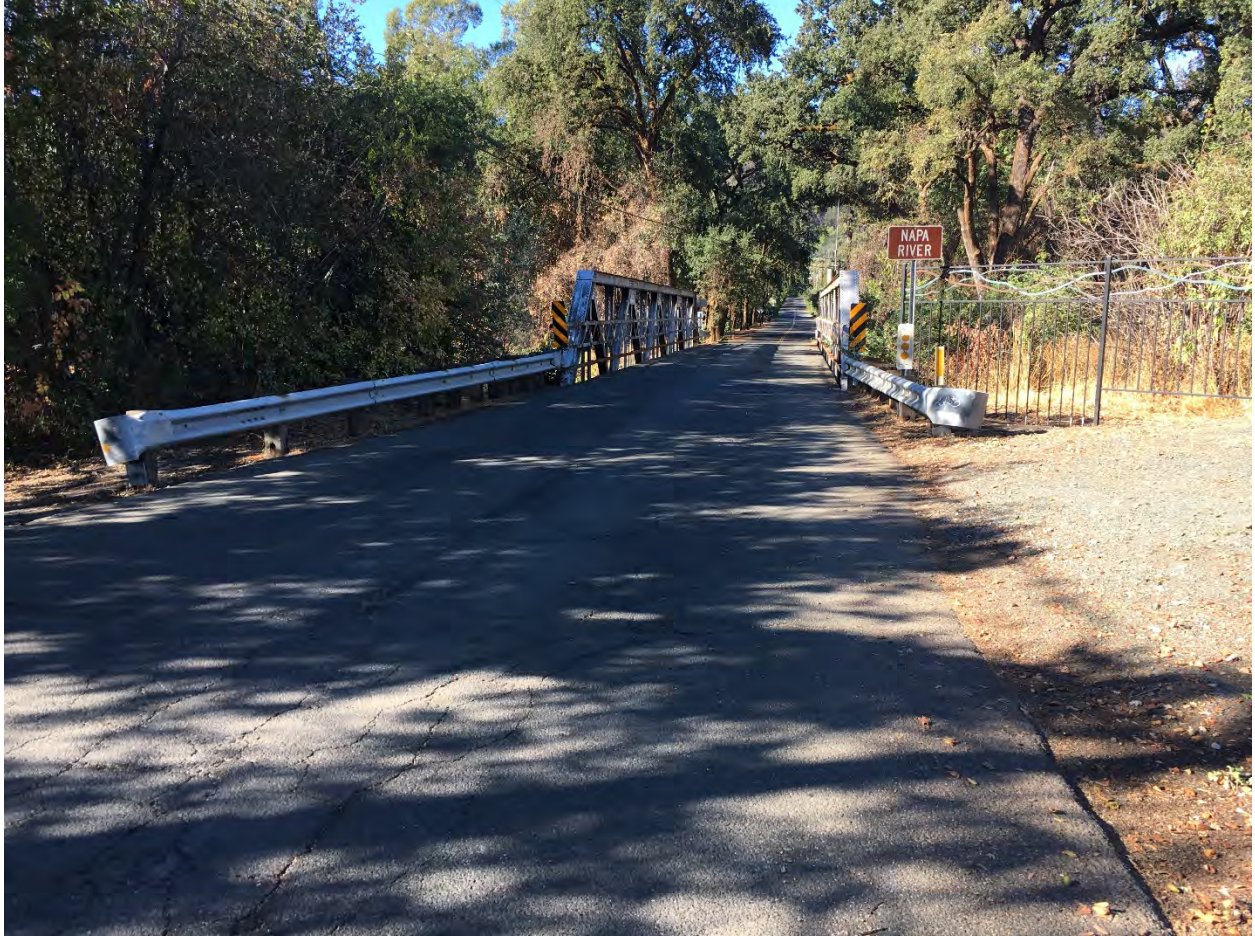
Photo #6: View of the Napa River bridge on Lodi Lane, west of the Duckhorn Driveway. Note taper and narrowness of the single-lane bridge.
