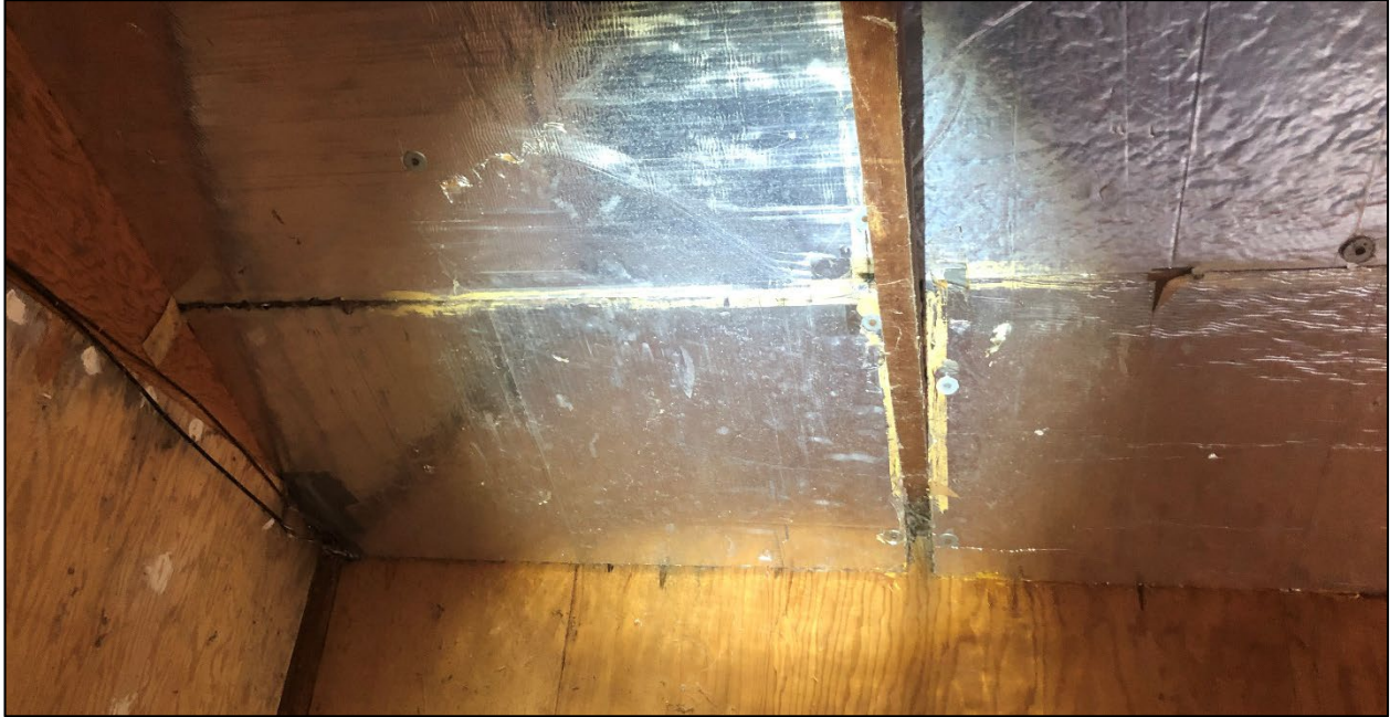
Photo 1: Looking at a typical section of roof inside the workshop. Insulation is held tight against the roof, eliminating interstitial spaces that might be occupied by bats. The workshop is also open with barn doors on either end that let in ample light and the area is regularly disturbed by workers.
