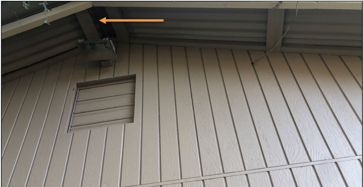
Photo 2: External roof and siding of the wine tasting/wine storage building. The metal roof is vented (see example marked by arrow) which eliminates any stable air traps that are necessary for bat roosting. The building is also sealed and regularly maintained for hygienic conditions to serve and store wine.
