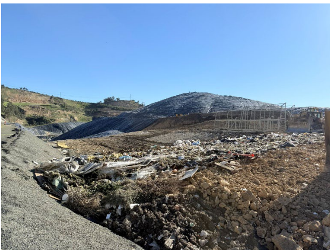
Module 5B- active filling area
