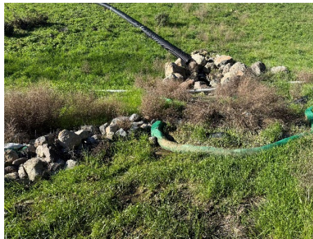
Stormwater conveyance outlet
