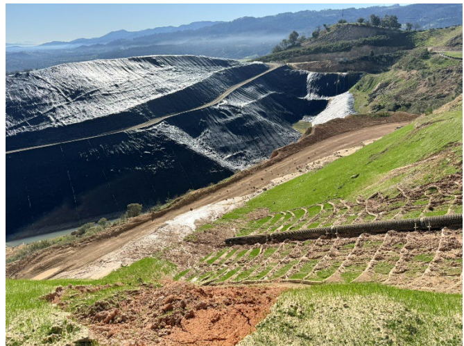
Toe of landslide, looking southwest
