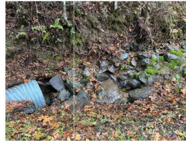
Photo 5: Culvert flow during precipitation.
