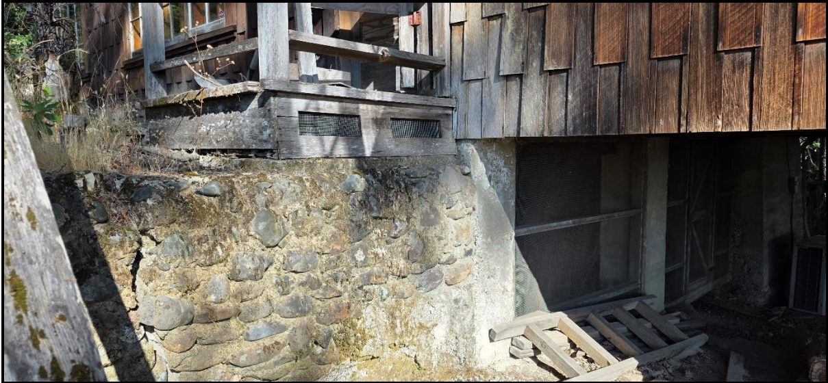
Figure 8. View of a portion of the basement and foundation of the large cabin.
