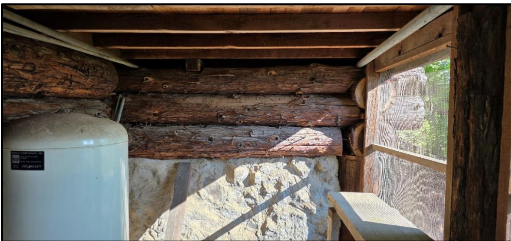
Figure 5. View of the basement area underneath the small cabin showing the retaining wall and foundation supports.
