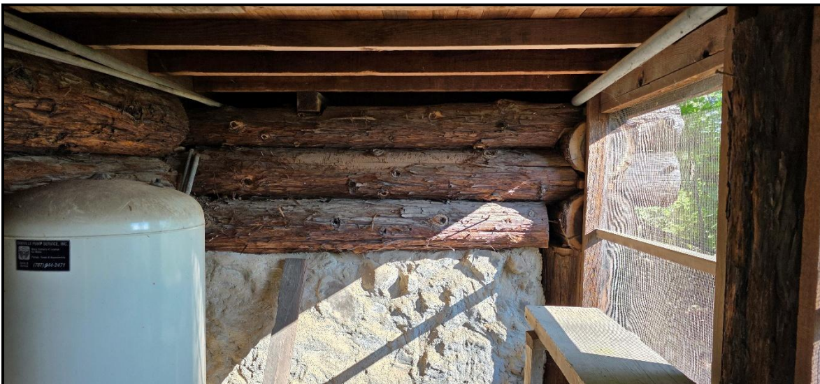
Figure 2. View of the basement area underneath the small cabin showing the retaining wall and foundation supports.
