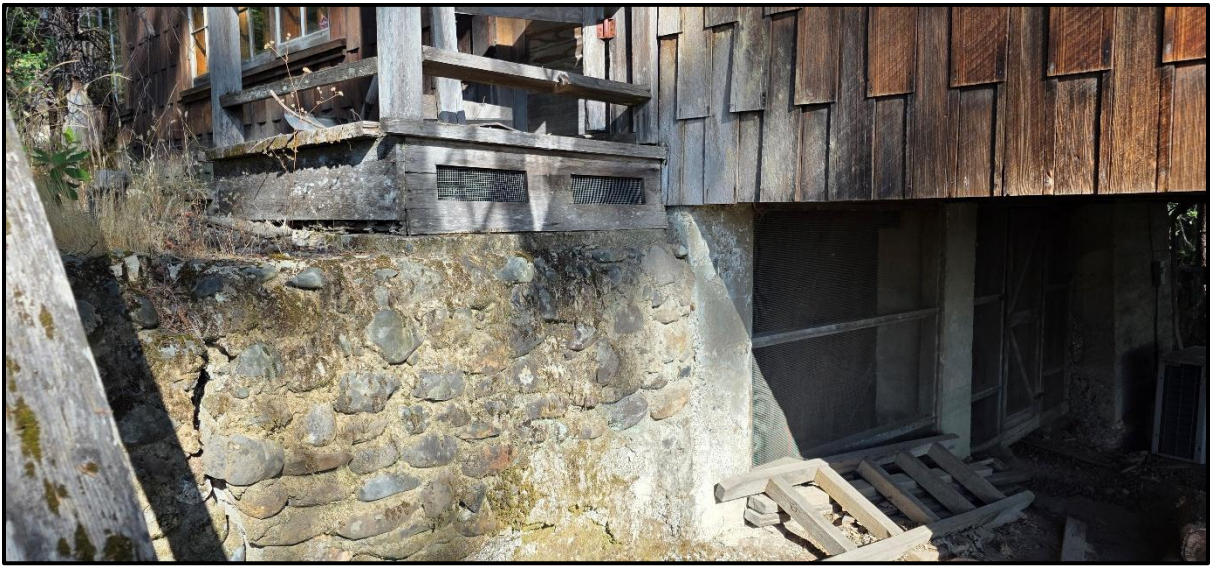
Figure 11. View of a portion of the basement and foundation of the large cabin.
