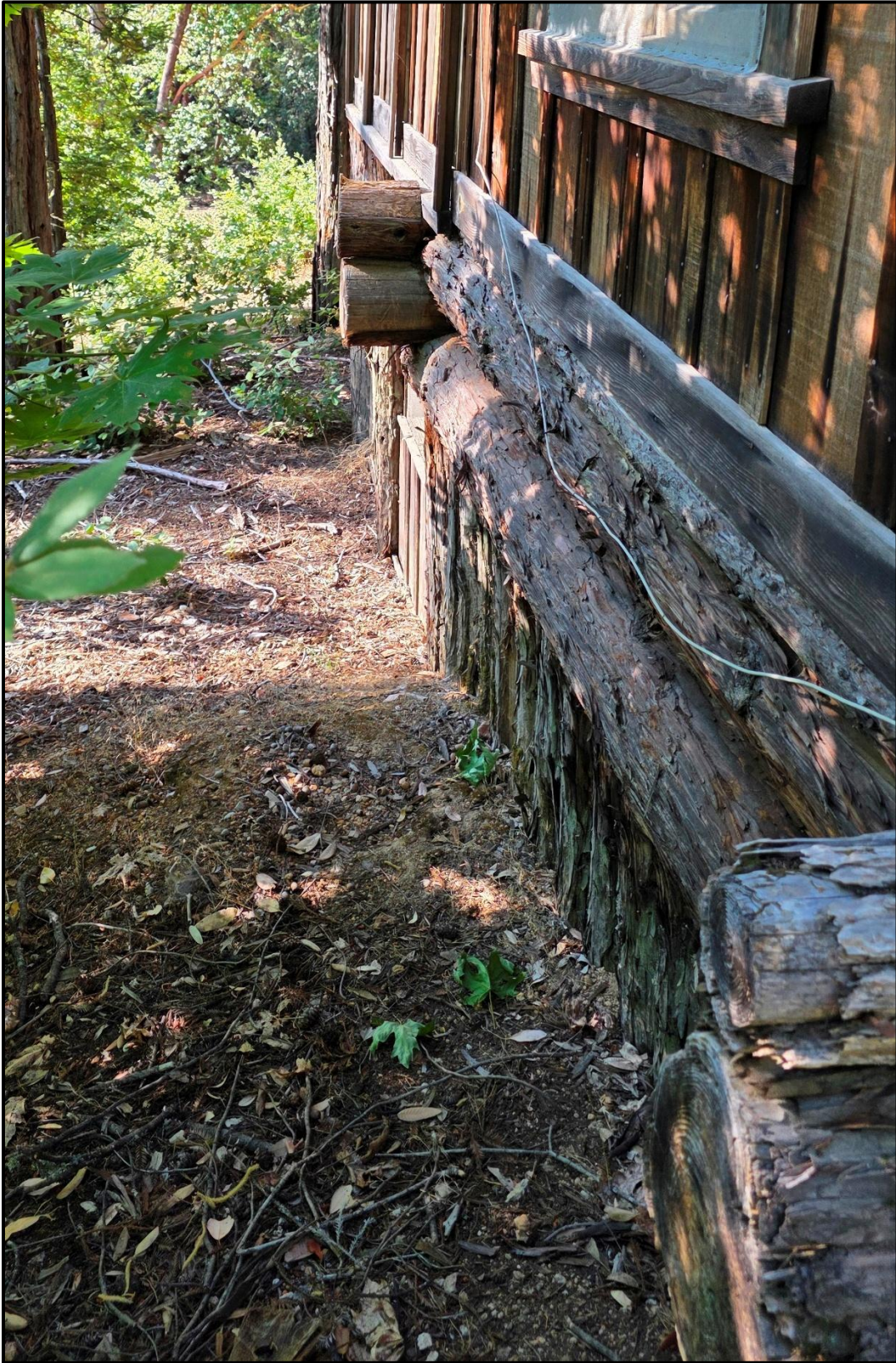
Figure 6. View of the east elevation of the small cabin showing the unhewn interlocking log foundation.
