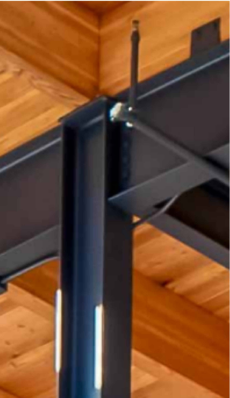
STRUCTURAL STEEL COLUMNS AND TRUSS
