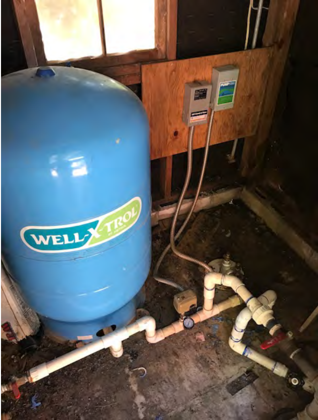
Well Site and Well Pump Equipment
