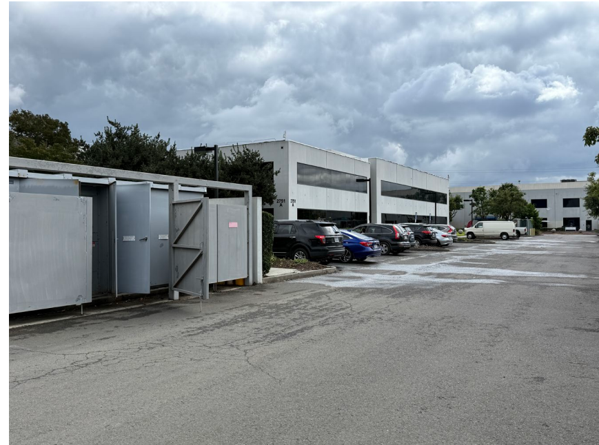
Bottom: Napa County HHSA parking stalls and electrical infrastructure
