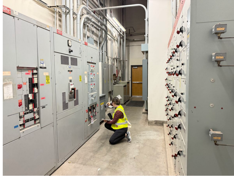
Top: CLEAResult Staff inspecting electrical equipment at Napa County HHSA Building
