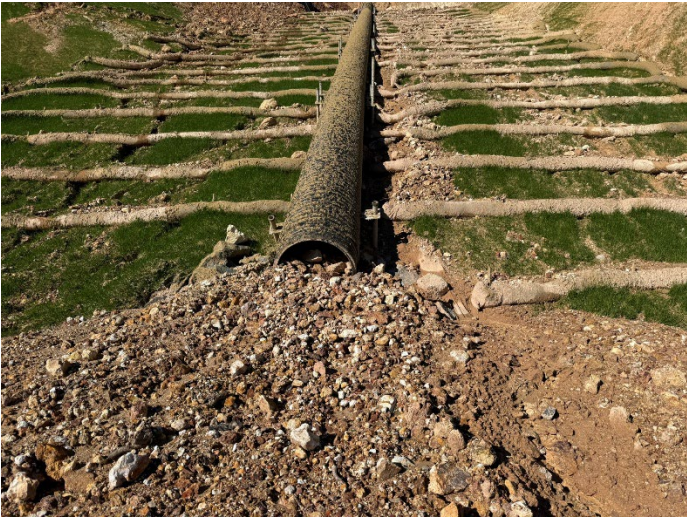
Stormwater pip below toe of landslide, filled with sediment
