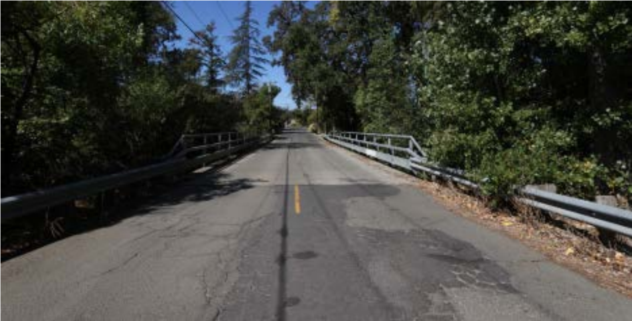
3D. No Pedestrian or Bike Facilities at Milliken Creek bridge
