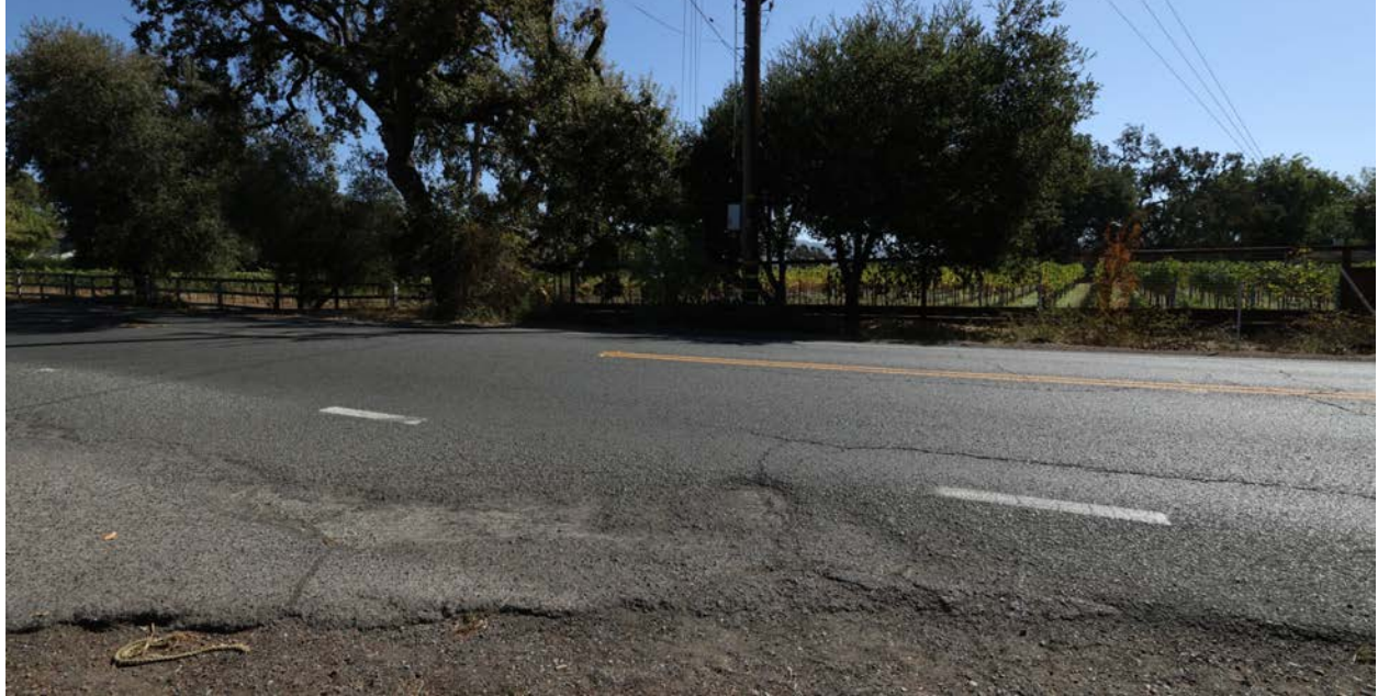
5B. Photo of Unprotected Left Turn on Monticello
