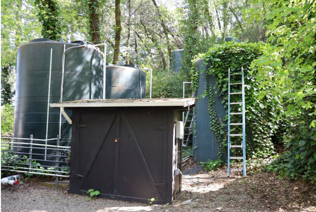
Figure 36. Five above ground water tanks and shed.
