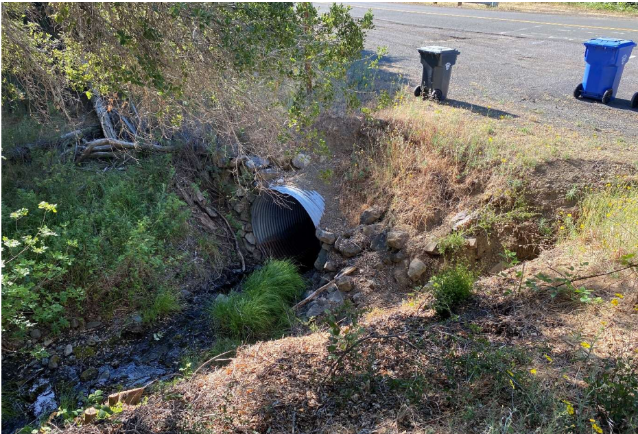
Photo 2. Inlet of the Dry Creek Road Culvert conveying flows from Campbell Creek to under Dry Creek Road.
