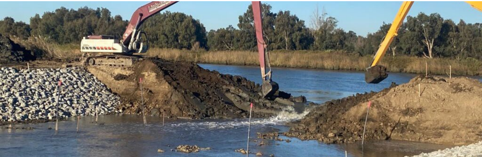
Levee breach in the Montezuma wetlands restoration project. Photo courtesy of the Montezuma wetlands project.
